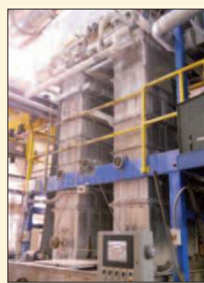
Aqueous Spray Cleaning Tanks & Risers
