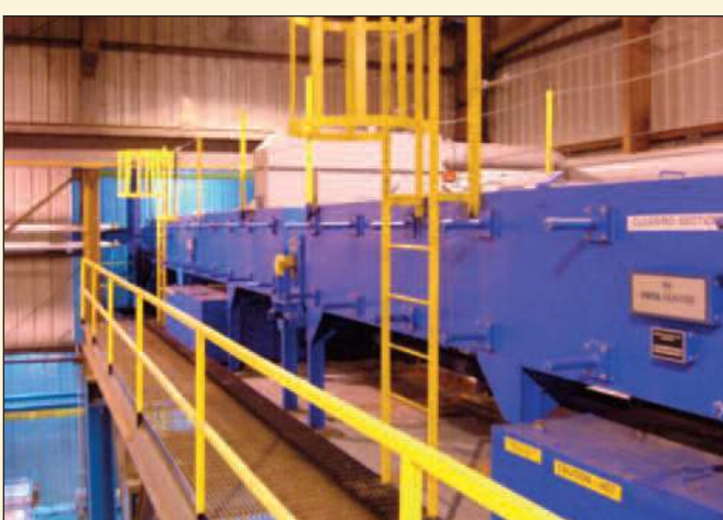
Wet Section, Second Stage Cleaning: (2) 29' Long Sections, 20 Spray Bars, 150 Nozzles, 660 GPM @40 PSI
