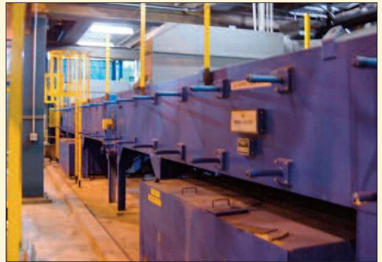
Wet Section, First Stage Cleaning: (2) 29' Long Sections, 20 Spray Bars, 150 Nozzles, 660 GPM @40 PSI
